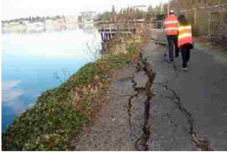
Figure 3-20: Example of lateral spread displacements causing cracking of pavement after an earthquake that occurred in Olympia, WA, in 2001 (after Bray et al. (2001)).
